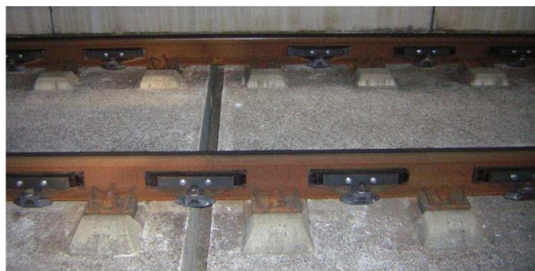
Rail dampers at the west track at section D2.
