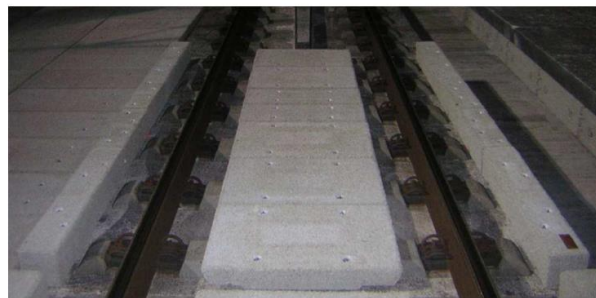
Absorption plates in between and next to the track at section D3.
